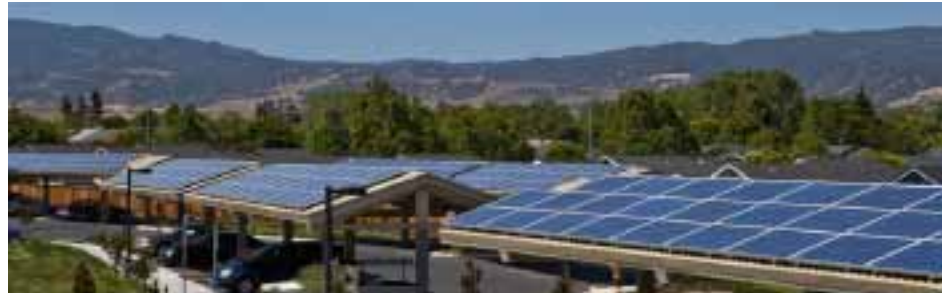
Vista Meadows Senior Apartment solar panels, Hollister, CA
